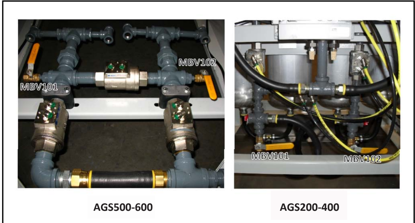
Figure 10: Manual Bleed Valves
